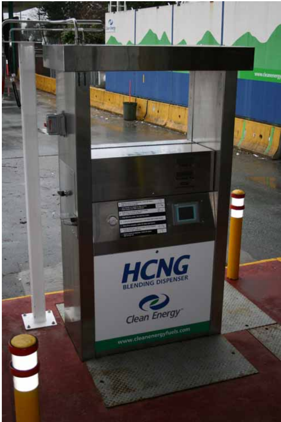
Figure 1.0 CNG/H 2 Heavy Duty Blending Dispenser Installed in Vancouver, Canada
